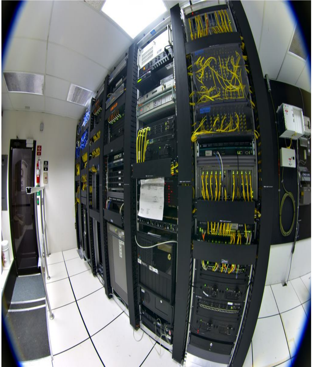
Fig.2.1:Example data center with cable tray installation
